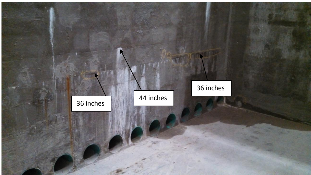
Filter #4 leak elevations measured from slab. (SW Corner)
