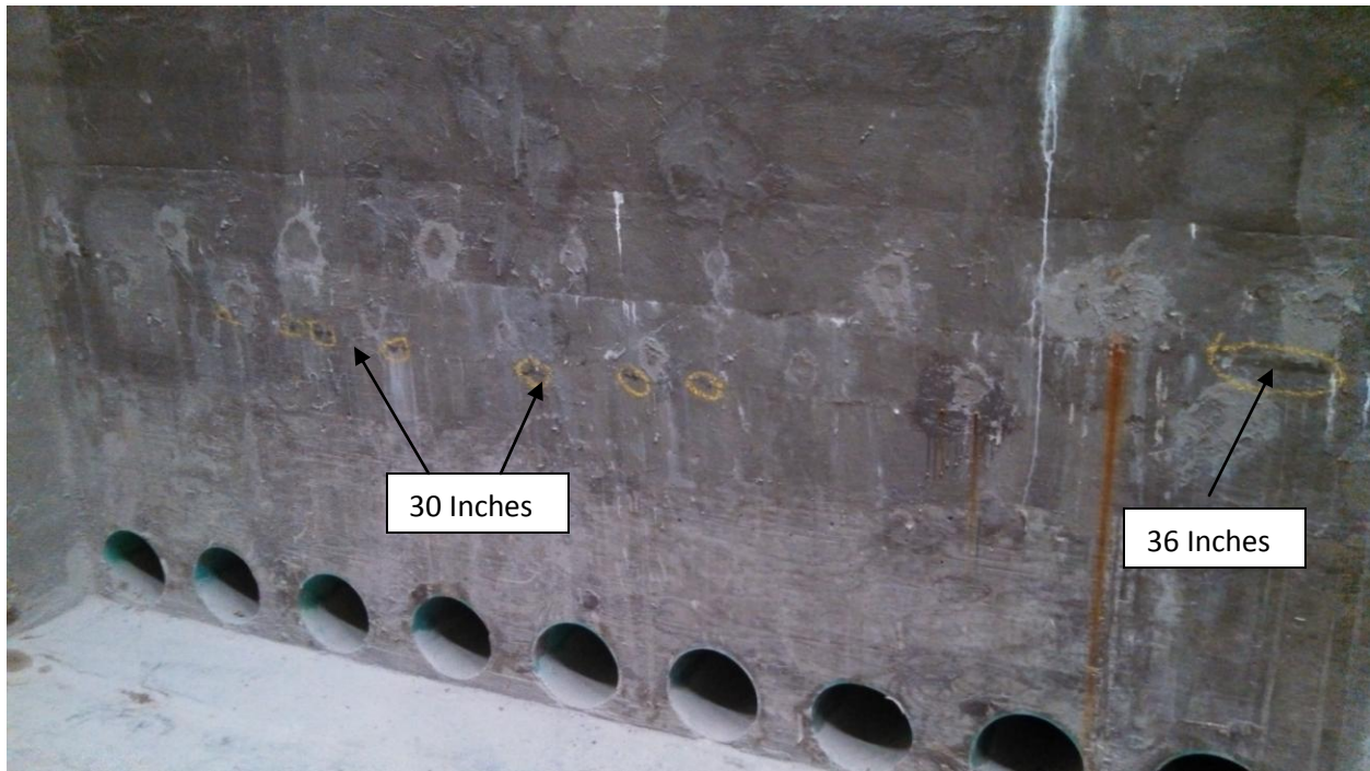
Filter #4 leak elevations measured from slab. (SE corner)
