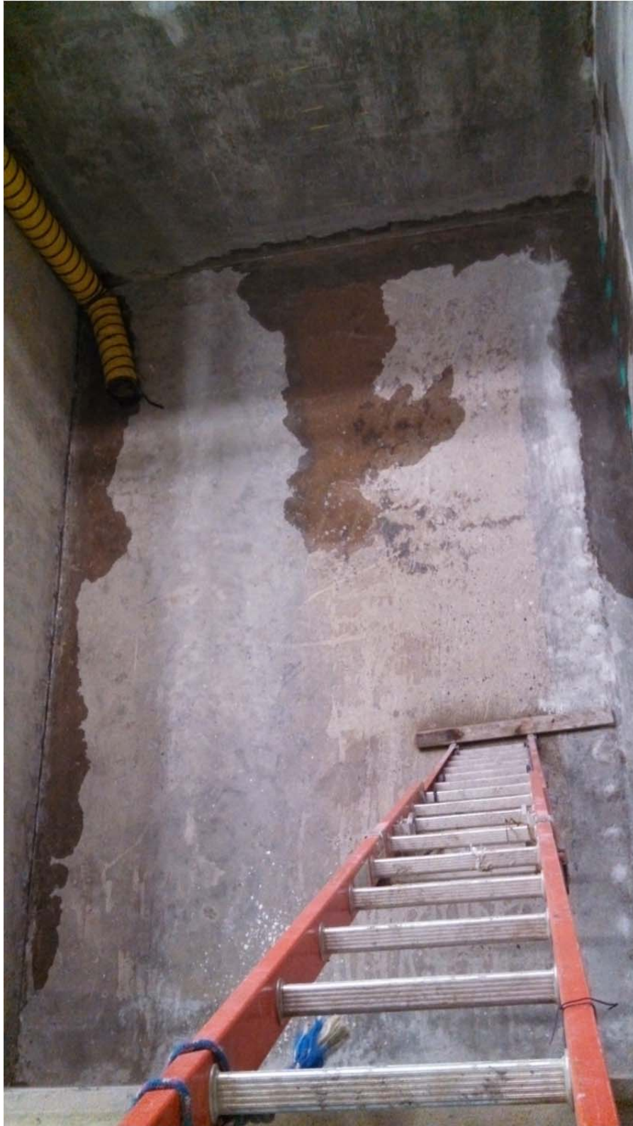
Figure 2. Pix taken by Al V 4/29/2014 w. 8 feet of water in F4. Shows influence on leaks in F3
