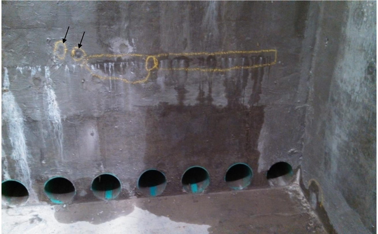
South wall and SW corner of Filter #4. Two small yellow circles on left side is where coating is blistering.
